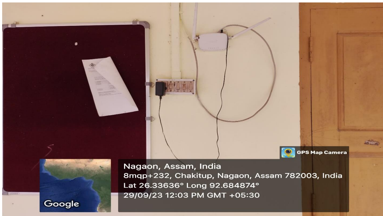
Internet and Wi-Fi Facility, new academy building
