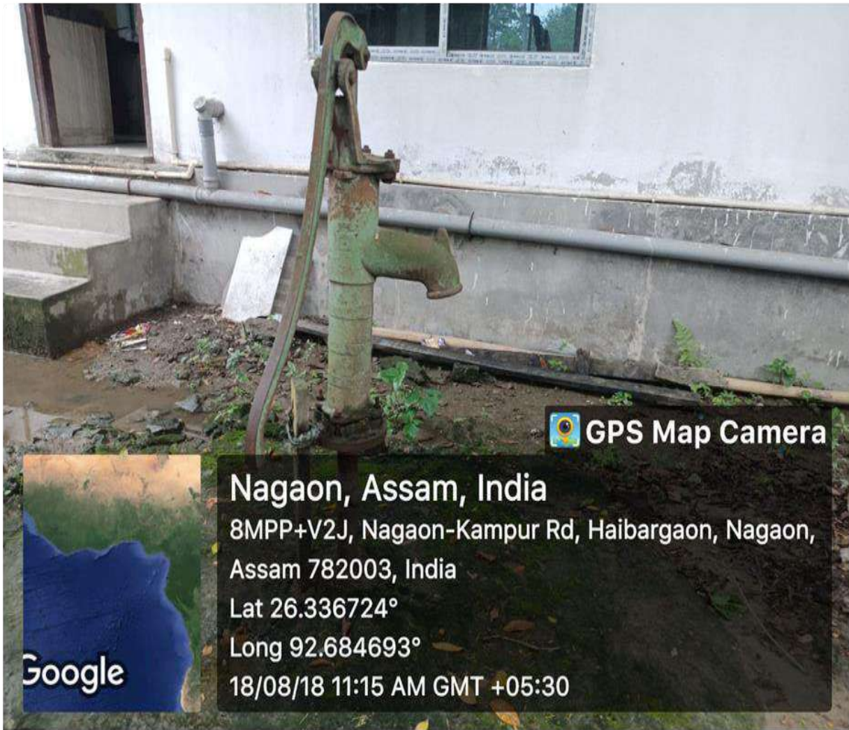
Figure 12: Photograph of the hand pump
