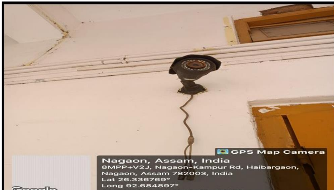
Figure 2. CCTV at different locations of the Campus
